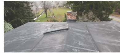
Abandoned roof hatch & North Chimney beyond
