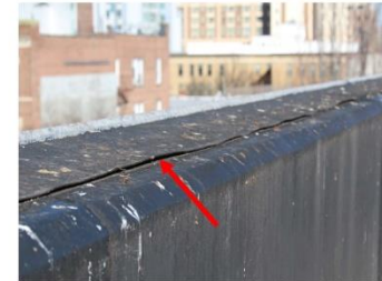
Photo 34. Open seams at parapet EPDM membrane.
