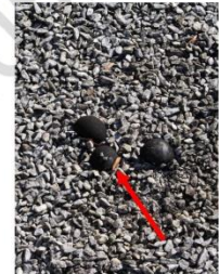
Photo 36. Detail of room membrane bubbling.
