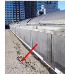
Photo 35. Roof membrane bubbling.
